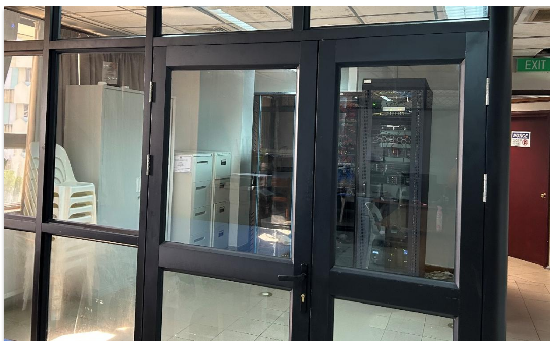
Figure 1The upgraded server room within the SBS Network Cabinet.
