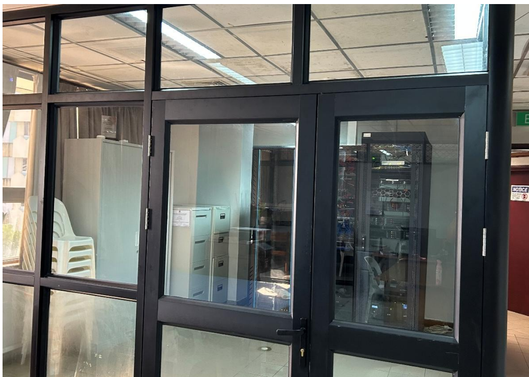
Figure 1: The upgraded server room within the SBS Network Cabinet.
